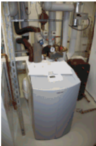
Figur 8.17: Varmepumpen for hele huset
